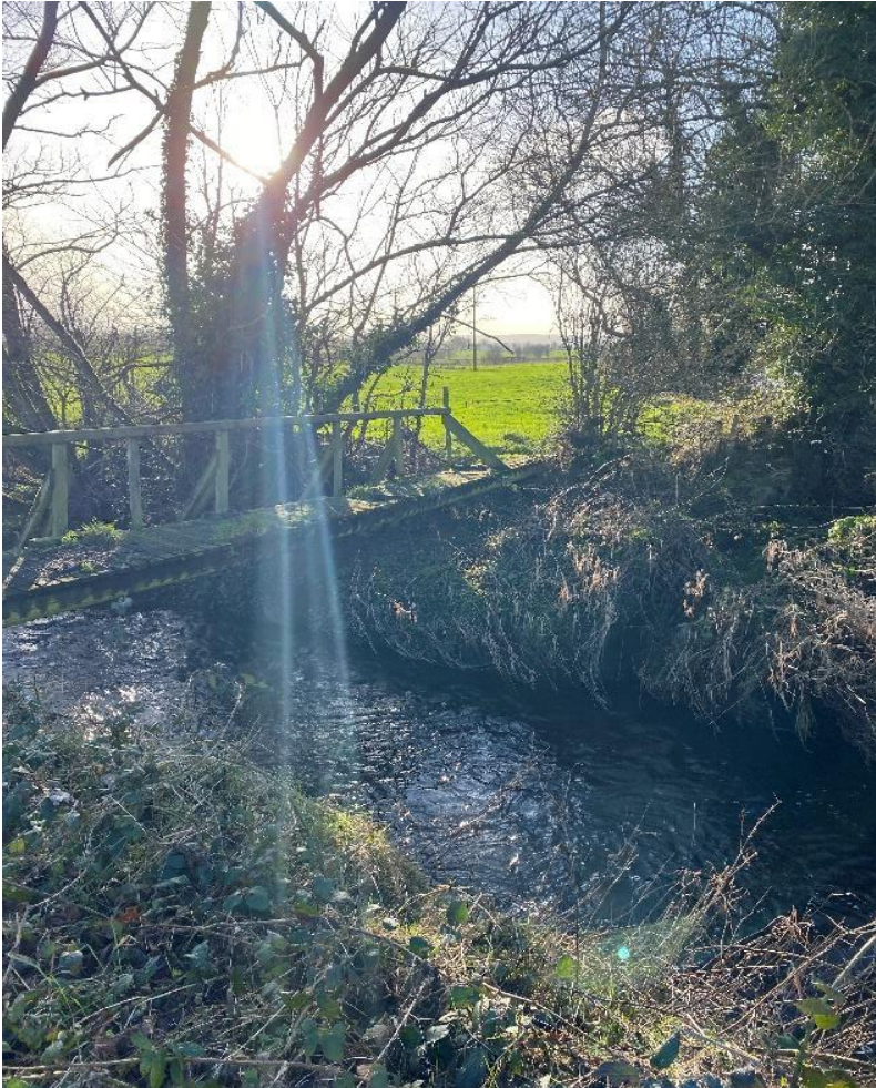
Figure 29: Footbridge degraded over time due to usage and weather.
