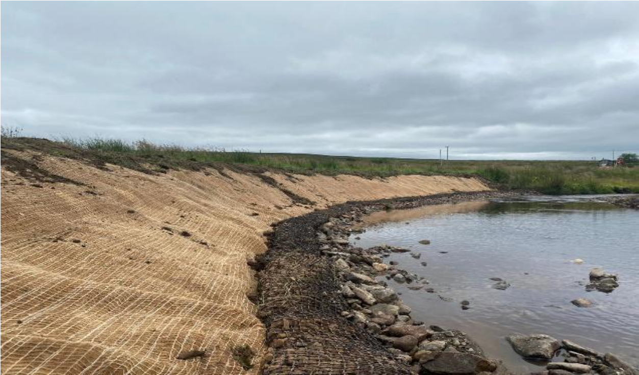
Figure 16: Additional Works implemented on the Elatagh included bank reprofiling of eroded and undercut banks.
