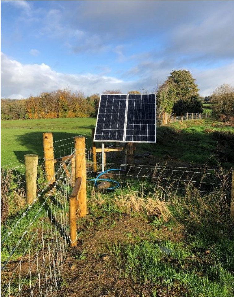
Figure 32: solar powered pump installed for livestock welfare.
