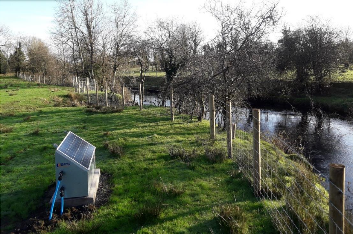
Figure 71: solar pump alternative water source for livestock.
