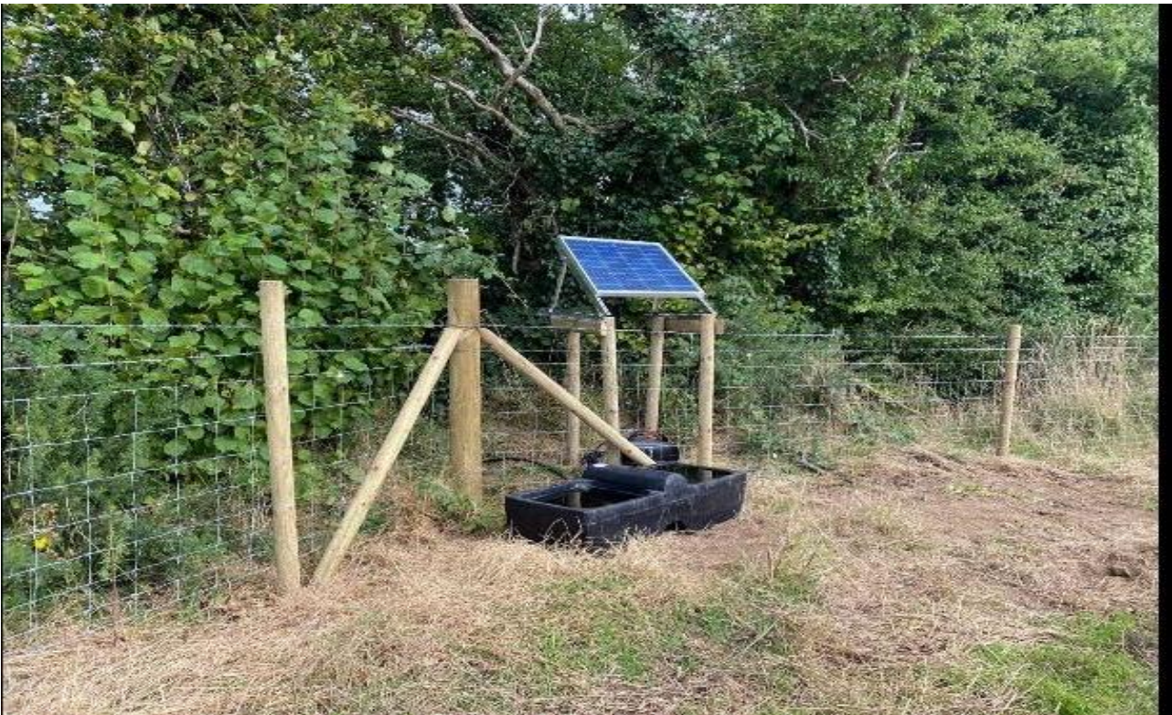
Figure 24: Solar powered pump and trough installed within the Dresnagh River Restoration works in lieu of preventing livestock access to the river.
