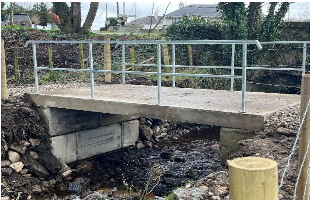
Figure 25: Clear span bridge replaced the potential barrier for landowner to access both fields on either side of river.
