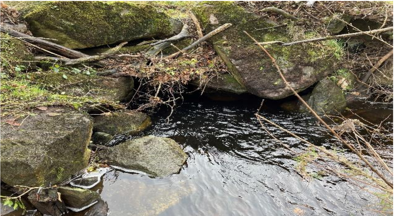
Figure 41: upstream view of the Rough Burn Barrier to fish migration.
