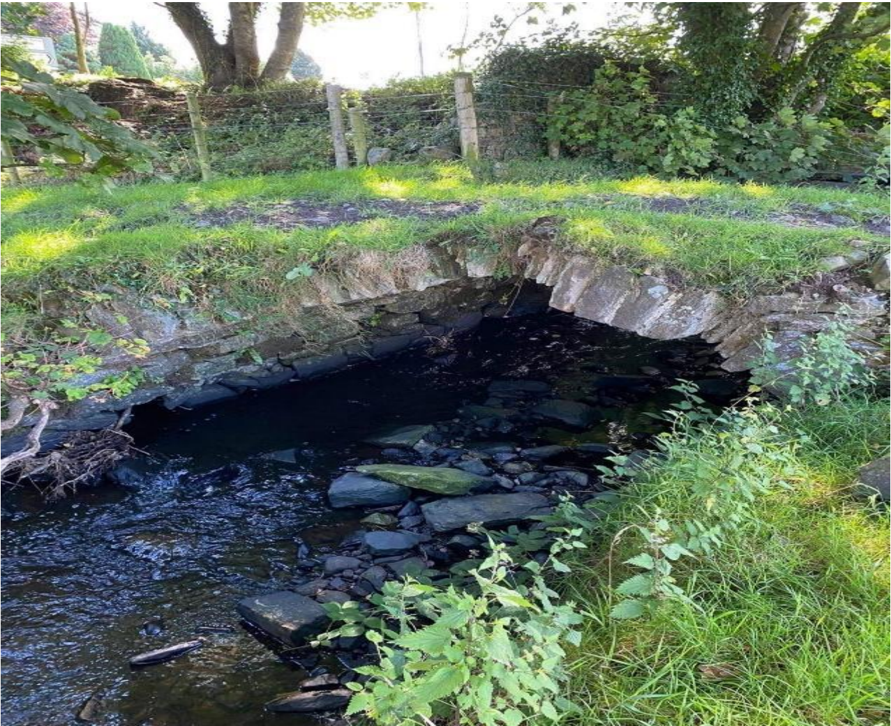
Figure 19: Bridge at risk of collapsing into river, causing a potential barrier to fish migration.
